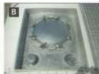
Manlid & pressure relief valve.
